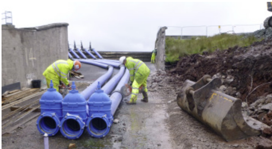
Series 01/79 gate valves being cut out of the temporary siphon lines for use on future projects.
