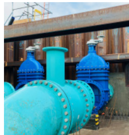
Series 54 reservoir-specification gate valves installed behind the siphon bulkhead.
