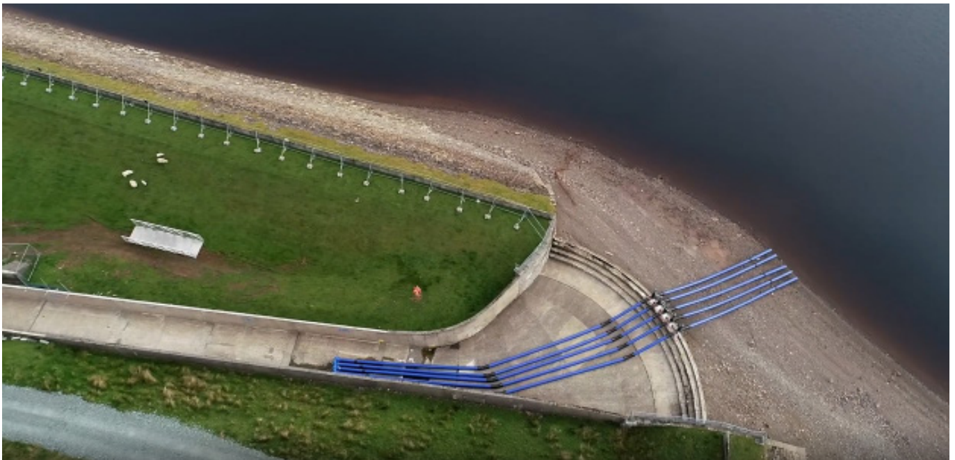
Aerial image showing the four temporary siphon pipes
